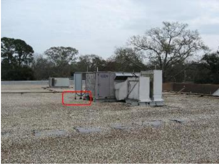
PHNS: Active Leak Area Main hallway of Programming
